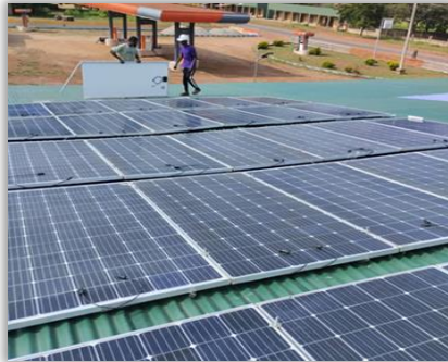
Shaybis Nigeria Ltd., Nigeria (IES) First of its kind Rice Mill in West Africa uses a 60kW Solar array to fully power rice processing machines
